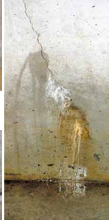
Leaking through cracks / joints
